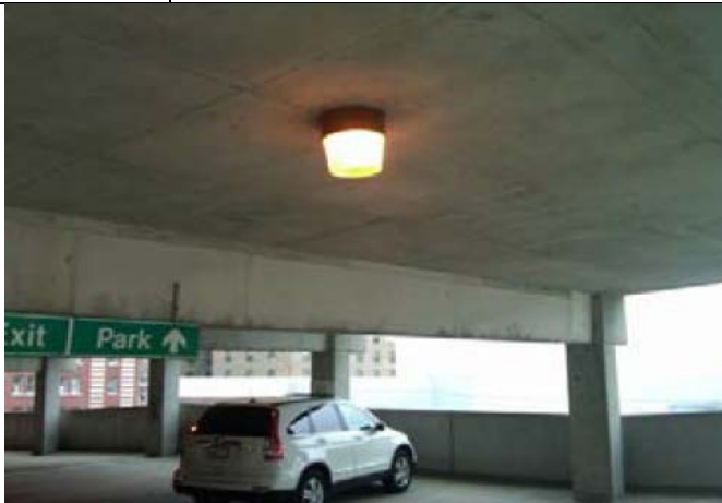
Description: Main Garage Lights All Levels
