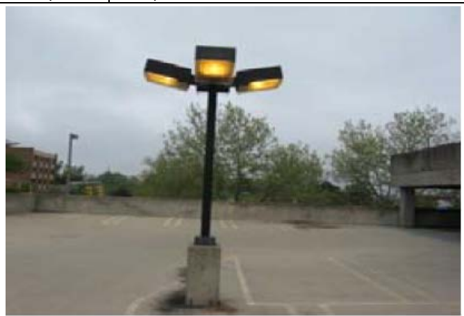
Description: Pole Lights
